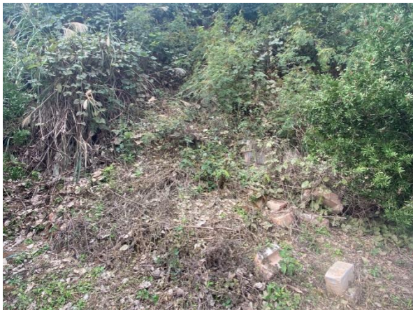
图 2 ZK4+684 左侧一级拱形护坡破损，S=5×6
